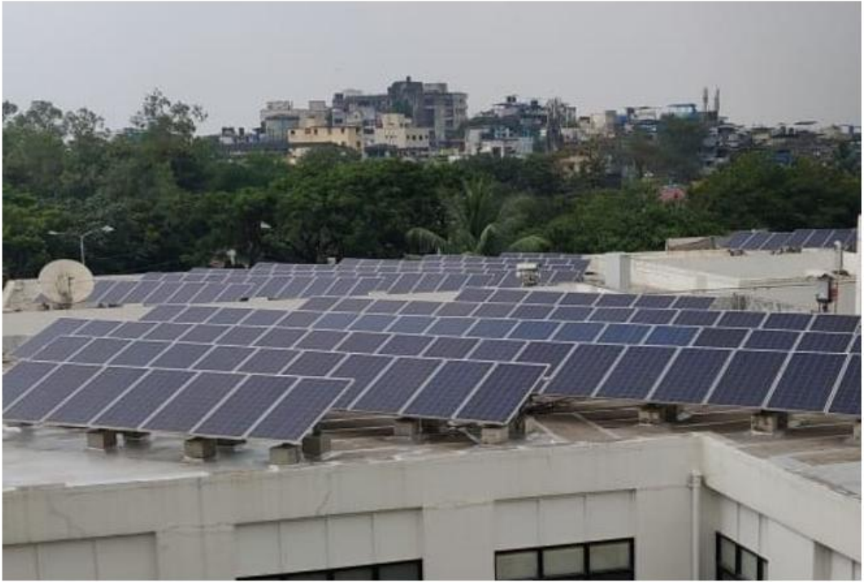
Rooftop Solar Panel System
